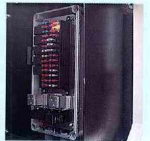
Faults detective electric system
